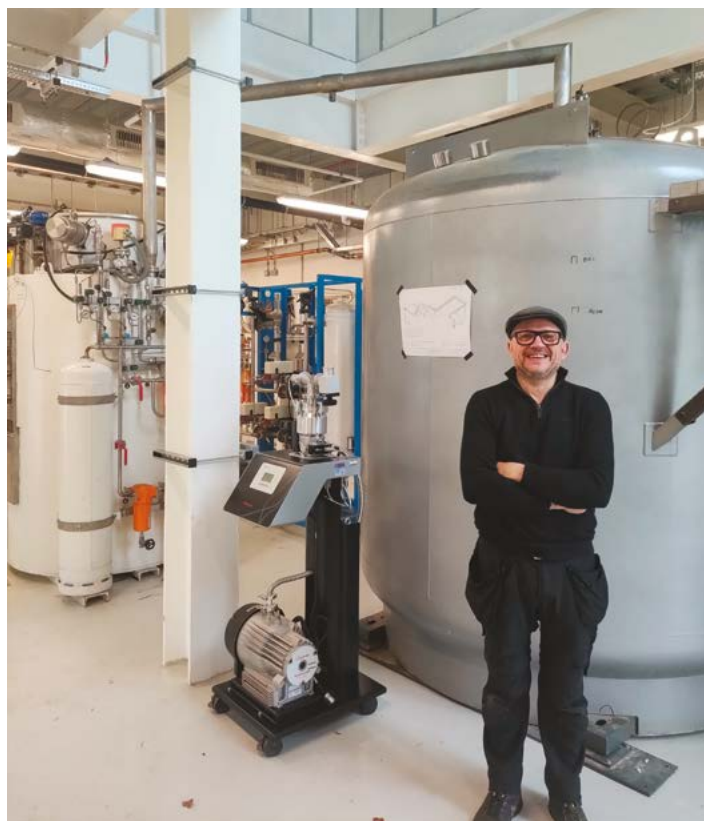
Dan Cross in front of the newly moved cryogenics facility at the Ray Dolby Centre.
